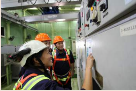
Specialised engineers maintaining machinery and systems
